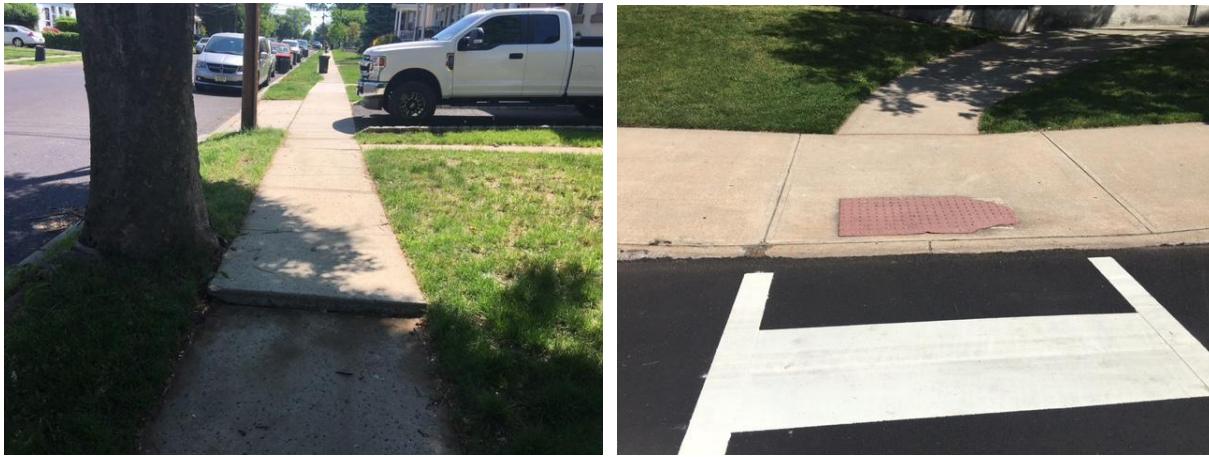
Uneven sidewalk on Second Avenue between Maple & Walnut Broken dome pad causing a tripping hazard near Lincoln School
